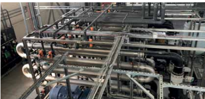
APATEQ deployed three HydraCell pumps within its five RO stages for processing leachate.
