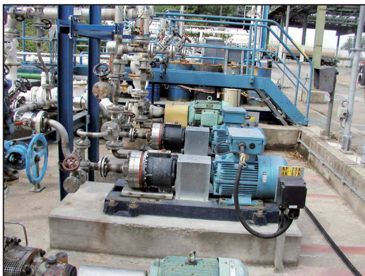
Figure 4: Low energy G35 pumps feeding polystyrol into distant process line
