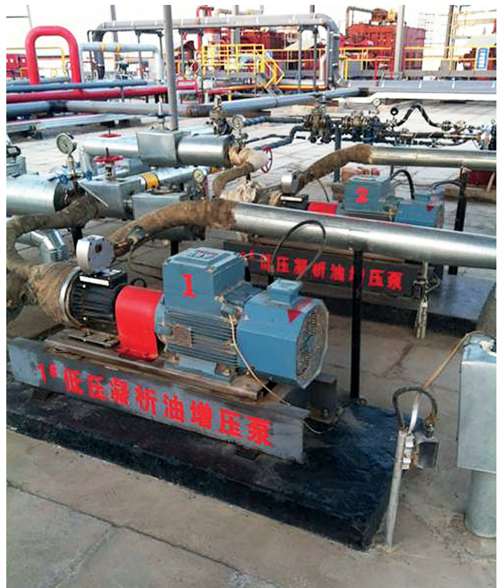
Hydra-Cell G25 replaced canned motor pump on transfer of gas condensate
