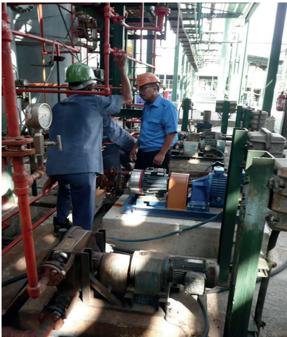
Methyl formate. Hydra-Cell pump and hose pump
