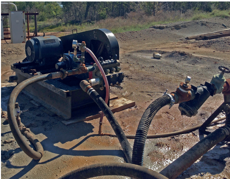
Leak-free injection of produced water at Texas oil well (T8045)
