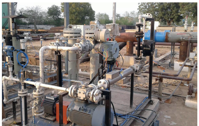
Figure 3. Hydra-Cell G10 and G15 sampling pump installations by Emerson Process Management (HPCL – Rewari Kanpur Pipeline network).
