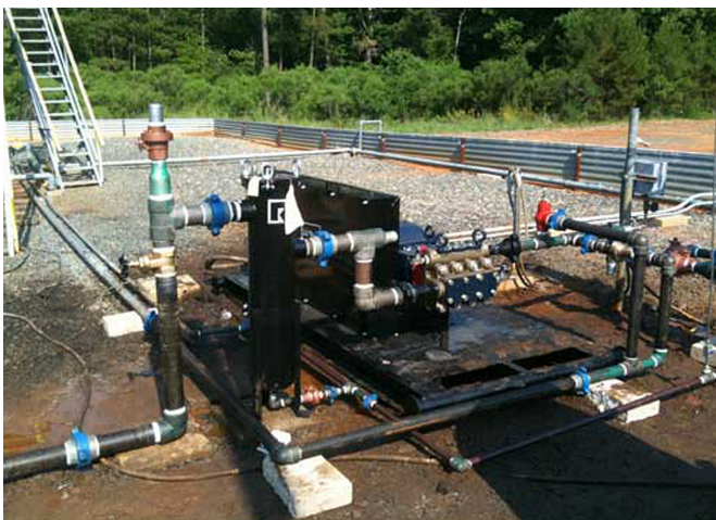
Figure 2. JJ Tech saltwater disposal system, with T8045 sealless pump.
